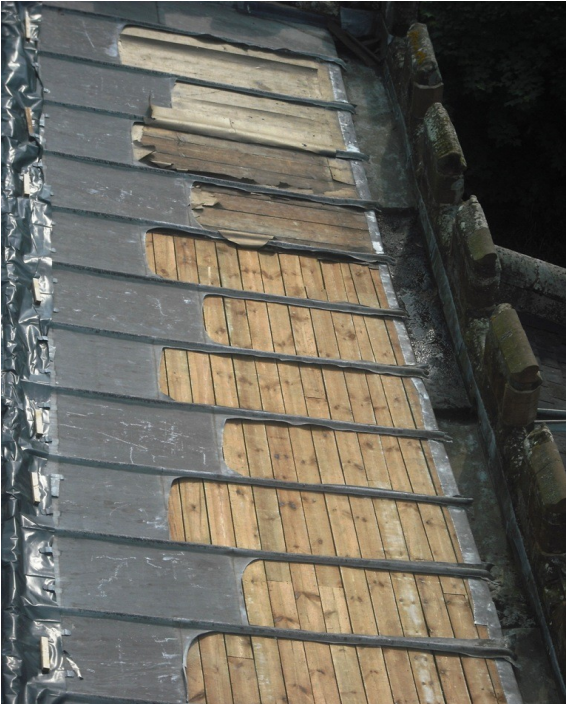
Church Roof showing missing lead
